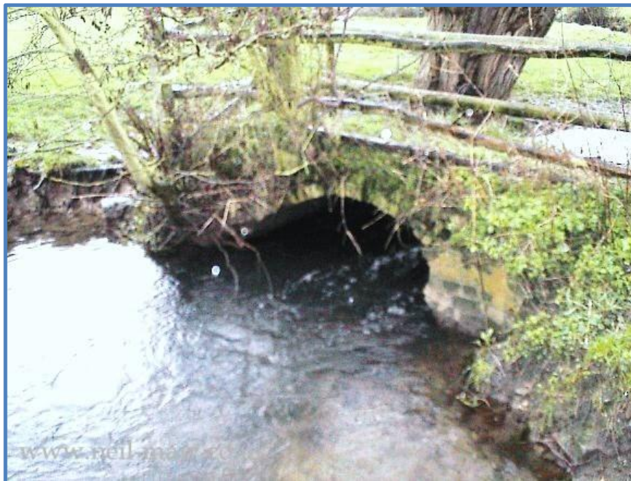
Above. The old 18th century Pennyhooks Bridge that was swept away by floods in 2004. Below. The splendid new bridge built by Neil Atkinson
